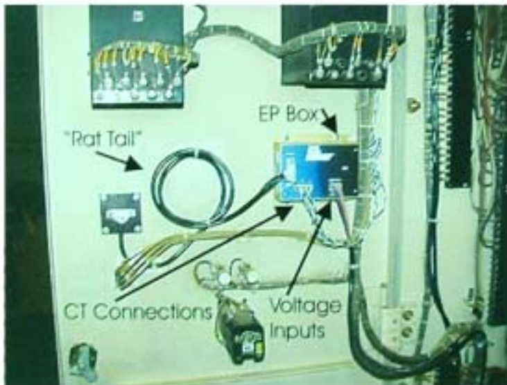
Figure3: Complete connection of EP in MCC Door.
